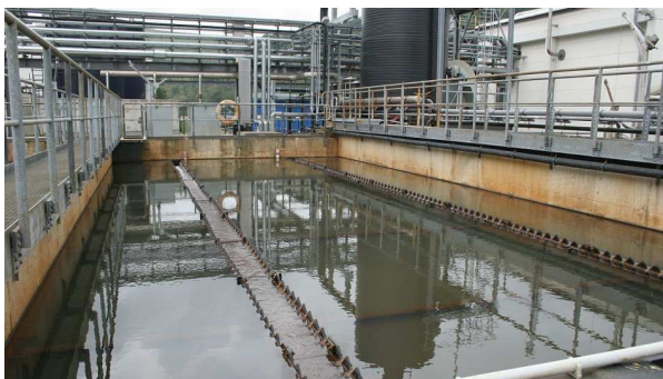
Fig. 1: Overview of the active treatment plant Schlema-Alberoda (Saxony, Germany) for the removal of uranium, radium, arsenic, iron, and manganese (2005-09-15, © Christian Wolkersdorfer).
